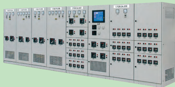
UPS REDUNDANT SYSTEM WITH DISTRIBUTION ACCORDING TO ENELPOWER SPECIFICATION FOR THERMALECTRIC POWERPLANT
